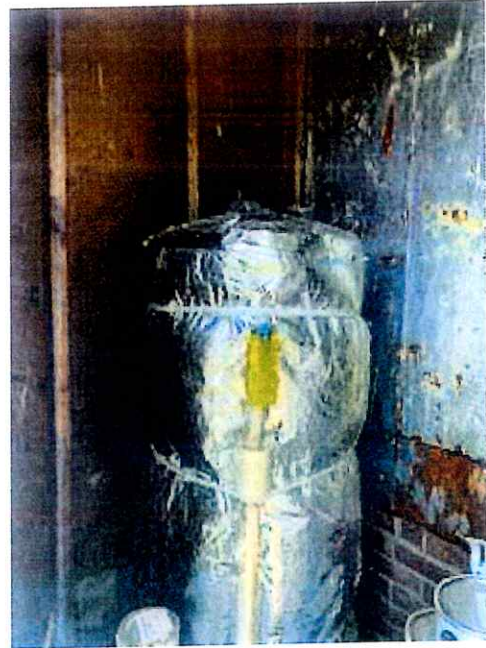
Pictured above is Hot Water Heater and Insulation that was completed by the Weatherization Team.
