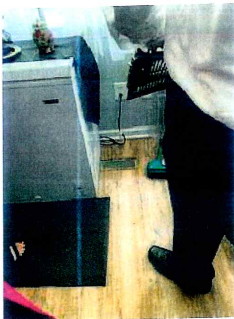
Mr. Bodrick removes the register, revealing the duct sealing.
