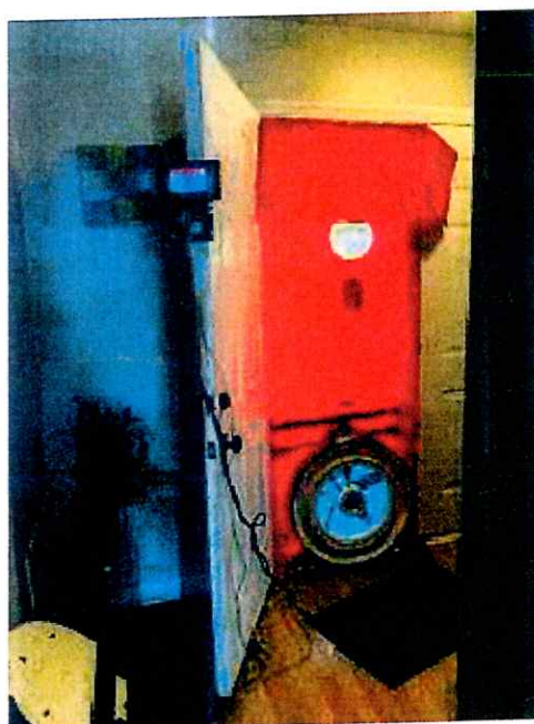
Blower Door tests can be conducted before and after air sealing to determine the effectiveness of the Weatherization Team's work.
